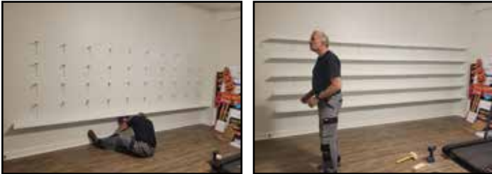
Above: Paul Stoner "measuring twice, cutting once," building and installing new shelves
